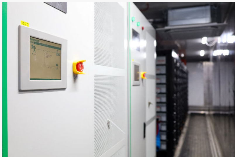
Wattstor battery energy storage system - an internal view of the container
